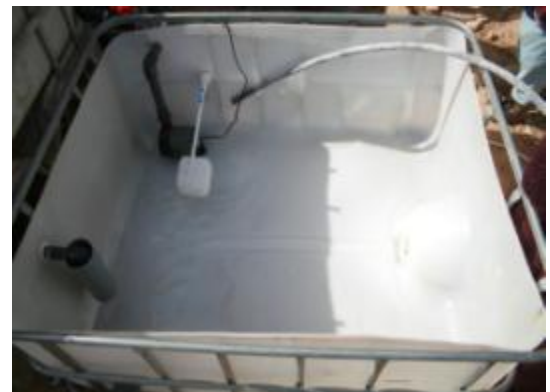
Figure 16: Raft/sump tank detail showing siphon drain pipe and splash guard (bottom left); pump plumbing assembly (top left) and ballcock valve (to the right of pump)
